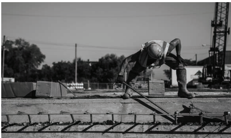
Zenith Tech employee stripping the concrete formwork from a freshly placed bridge deck on Capitol Drive, City of Milwaukee, N. Green Bay Avenue to N. 2nd Street.
