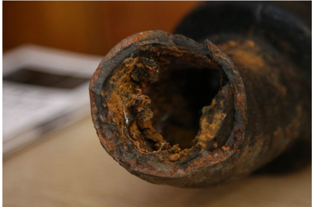
Lead Water Pipe Photo: WSJ
