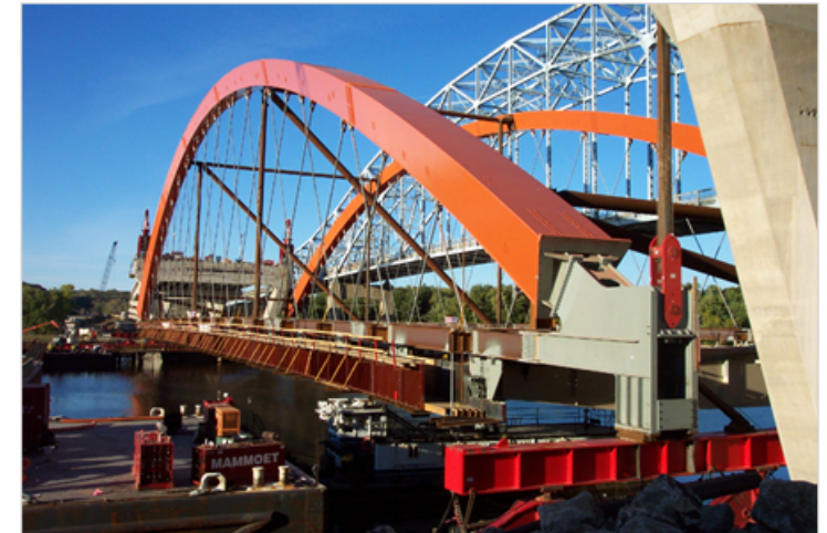
The Hastings Bridge replacement Main Span was constructed off-site and lifted into place from barges in the river.
